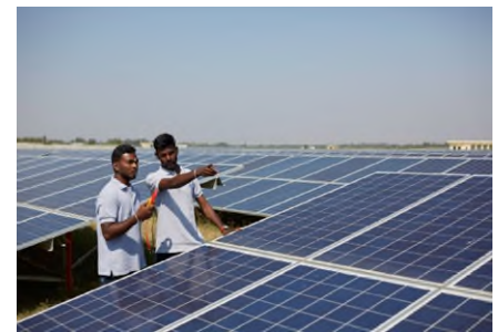
Clean energy technologies as this solar plant in Bevinahalli, India, already offer considerable employment potential. KfW Photo Archive / Dawin Meckel / OSTKREUZ
