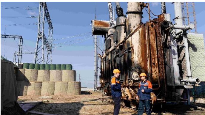
Employees of Ukrenergo in front of a transformer hit by a drone in central Ukraine. Image source: KfW Bildarchiv / Jonas Wresch.
